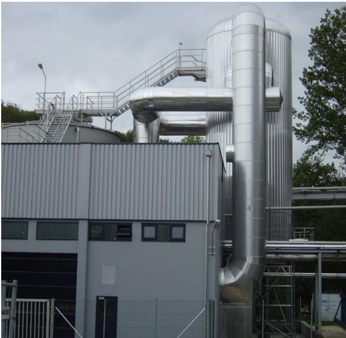
MVR Plant in the Sulfite Pulp Industry
